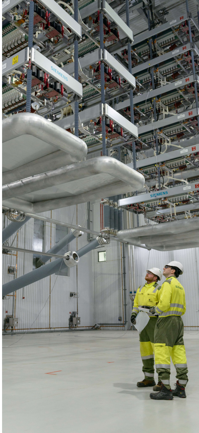
Image: SP Energy Networks Western Link valve halls.
